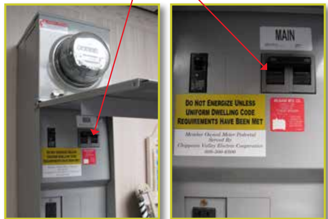
Lift meter pedestal cover to find breaker
